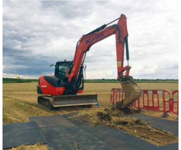
Photo: The digging of a trial trench from the recent Site Investigation campaign.
